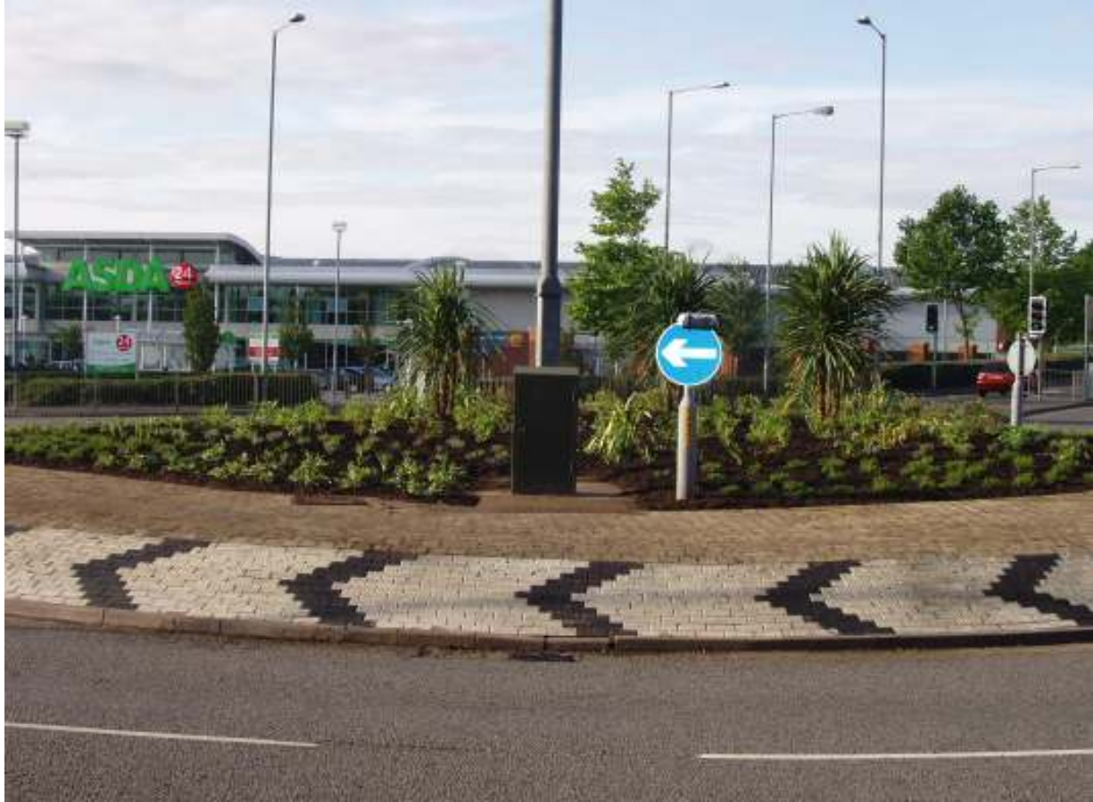
All works completed in five days working between the hours of 18.30 – 21.30 with full traffic management supplied by our fully trained staff
